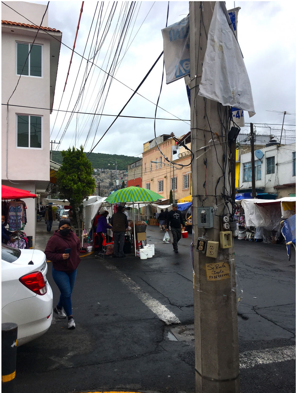
Improvised electric sockets hooked to public electricity in a neighborhood tianguis. Photo credit:
