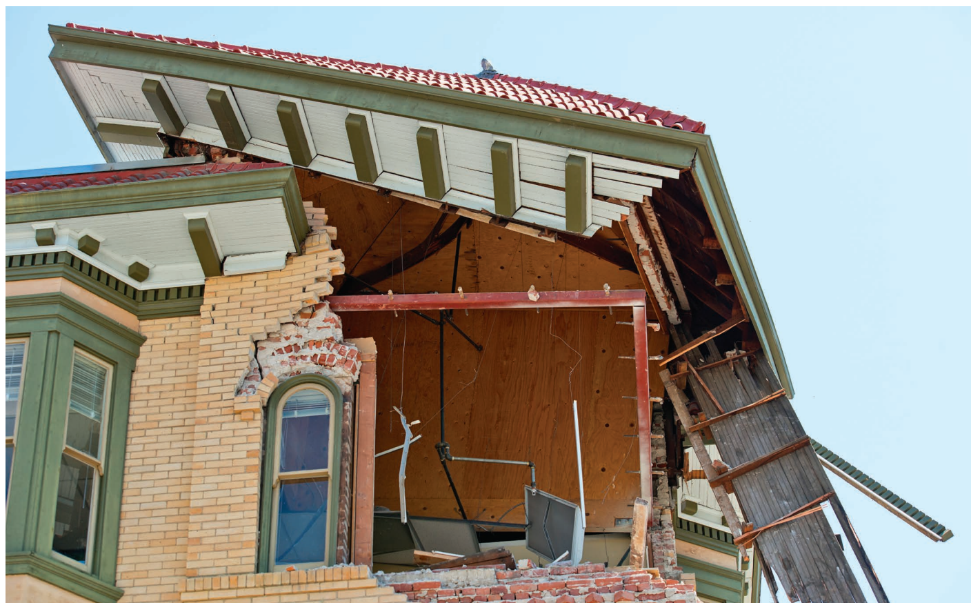
Damage from the Napa earthquake of August 2014.
